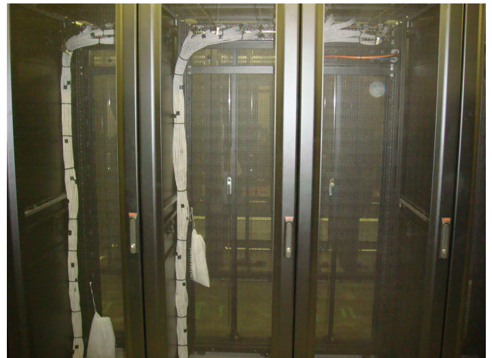
Each server rack was equipped with a 48-way Category 6 copper cable link going back to the main comm's row
