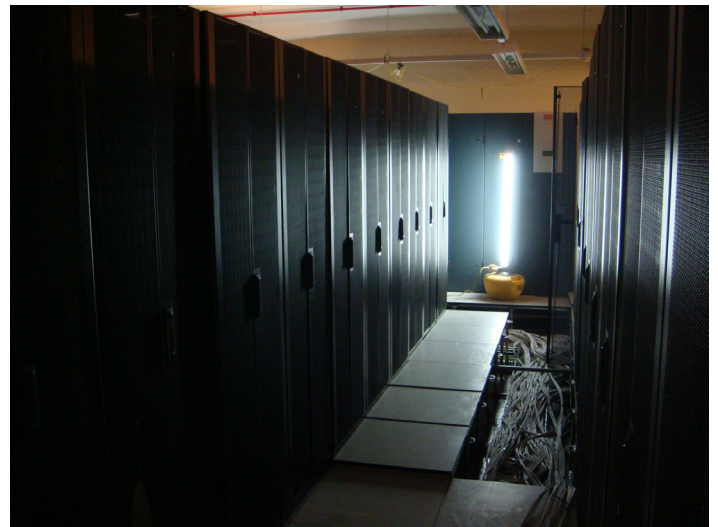
Tier 2 data centre with 48 server racks and ten comms racks plus an entrance facility housing another five comms racks
